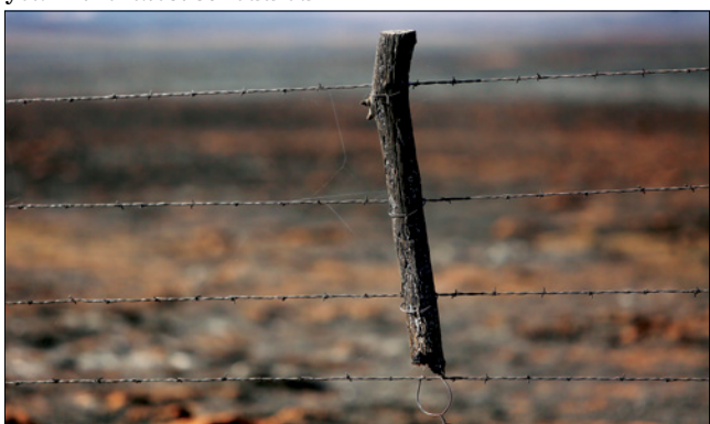
Burned fencing lines U.S. 160 near Ashland on Thursday.
